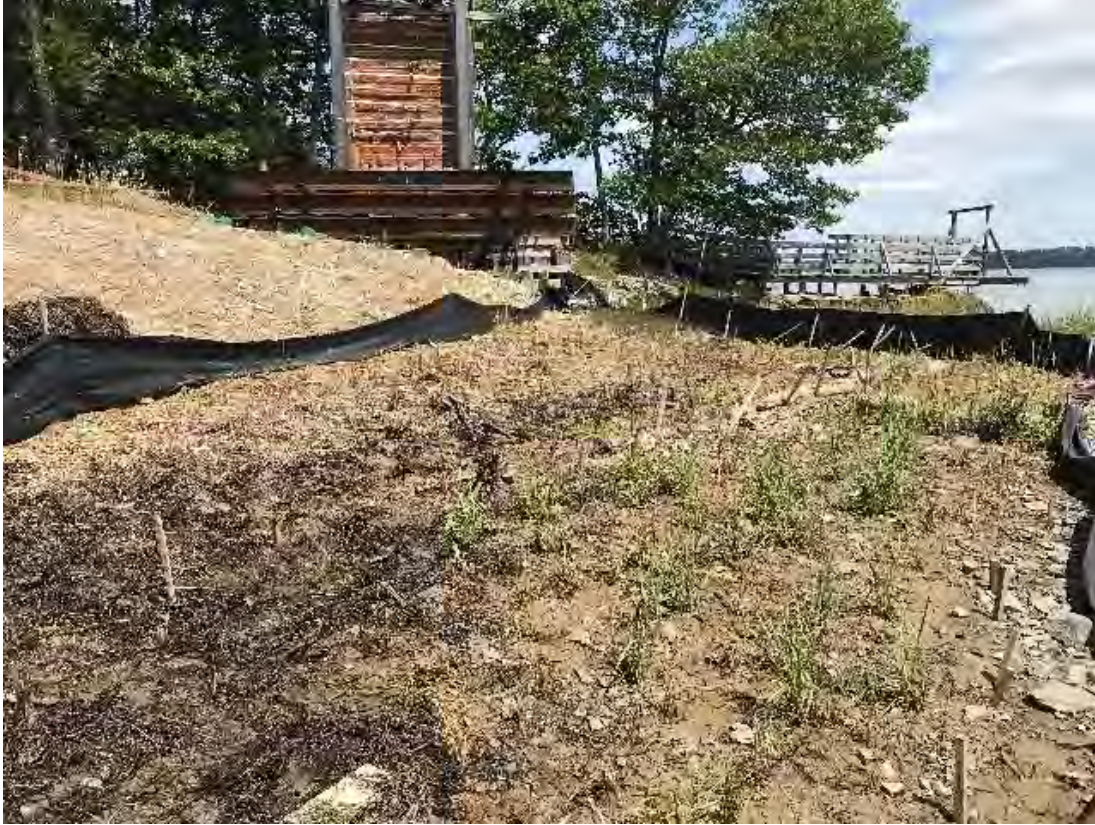
Fig 17: Salt marsh restoration and cable house in background at Eversource property/west side of the bay. Viewing north (07-27-20).
