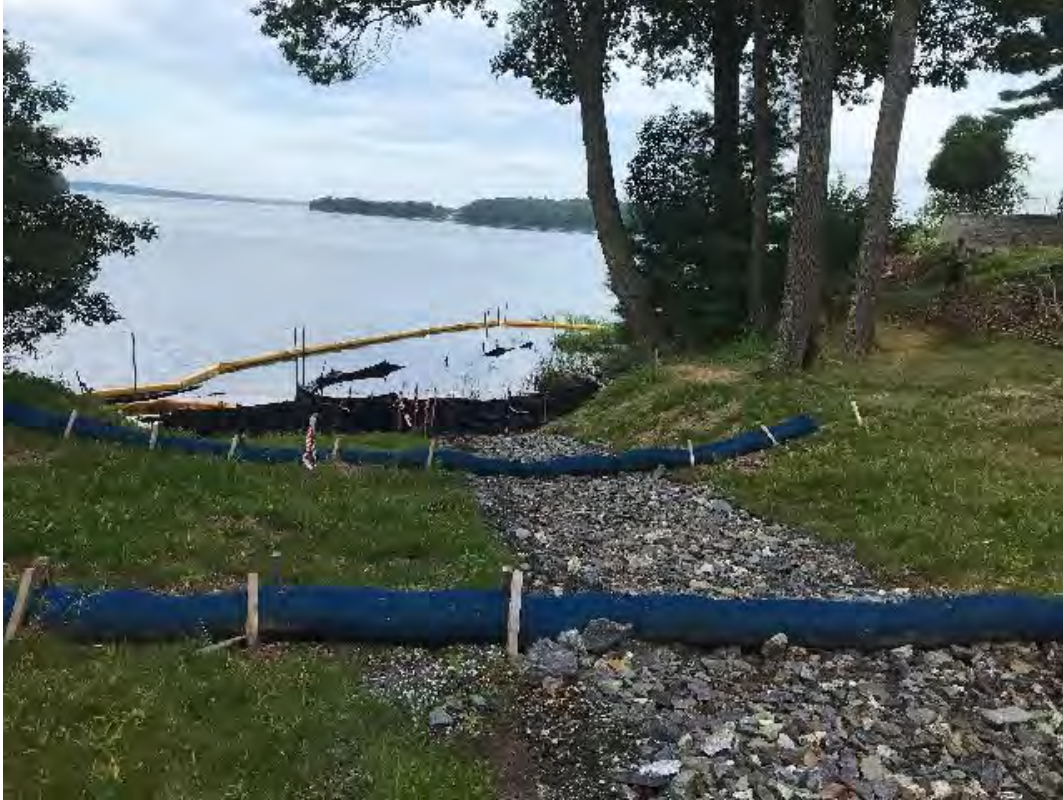
Fig 15: Slope below manhole at Gundalow Landing/east side of the bay. Viewing west. (07-27-20).
