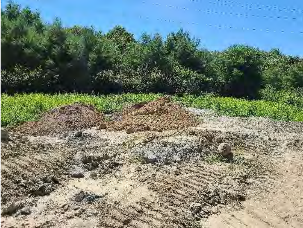
Fig 11: Soil for turtle nesting area, sourced from dewatering basin at Str. 48. Viewing south. (07-29-20).
