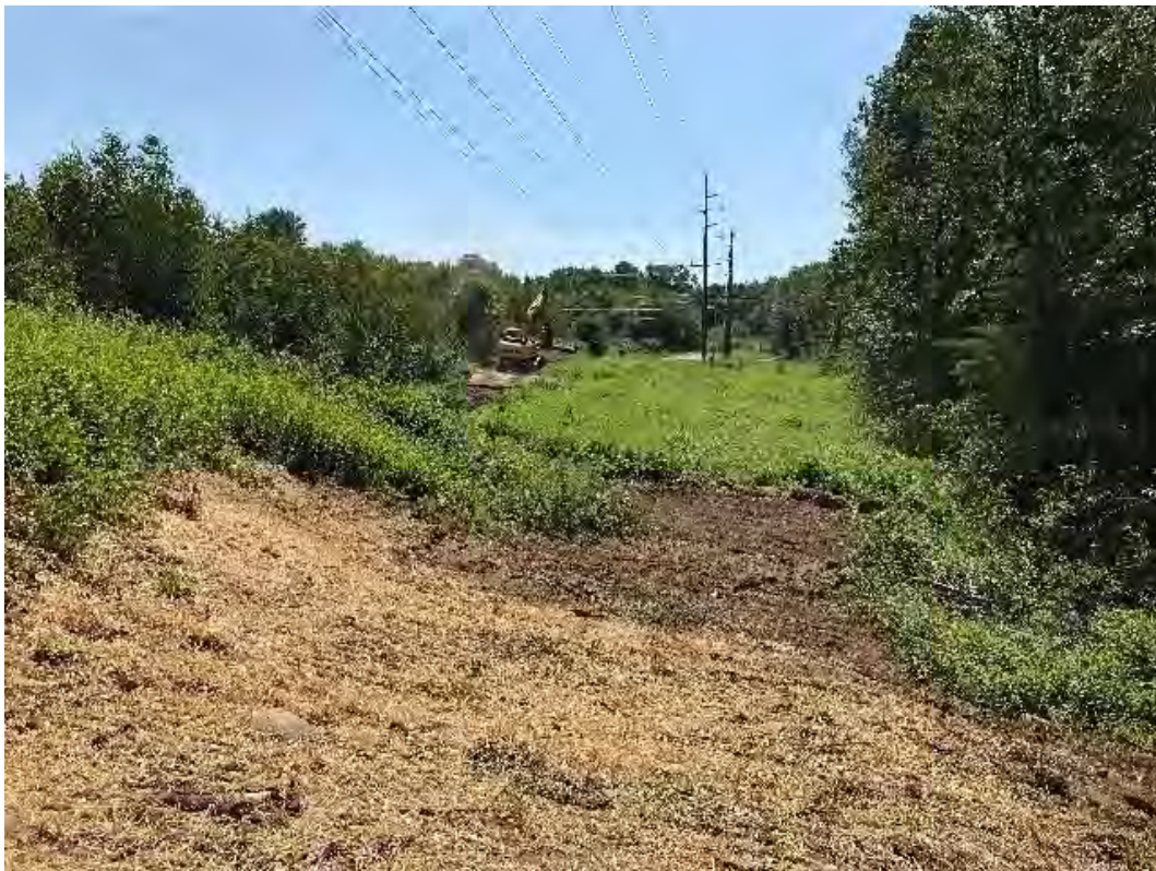
Fig 4: Access road leading to Str. 47 from Str. 46 in process of being restored. View south. (07-27-20).
